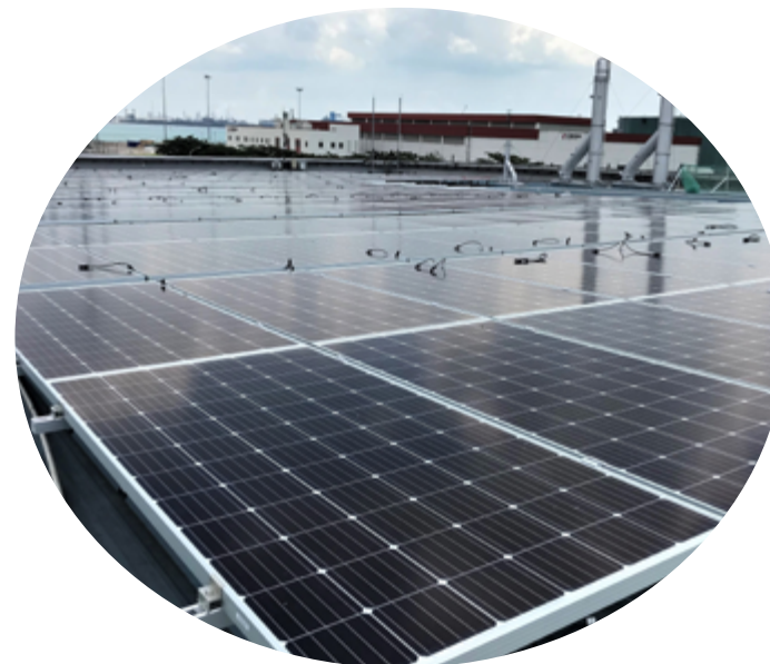
Photo: The solar energy project at our Tuas Mill in Singapore is the first Kimberly-Clark onsite renewable energy project in the region and is one of the largest solar panel installations in Singapore.
